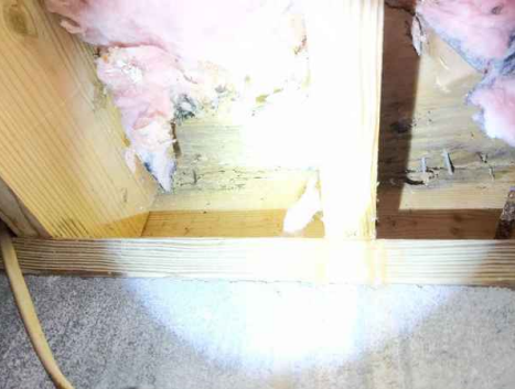
4 - below the front door
