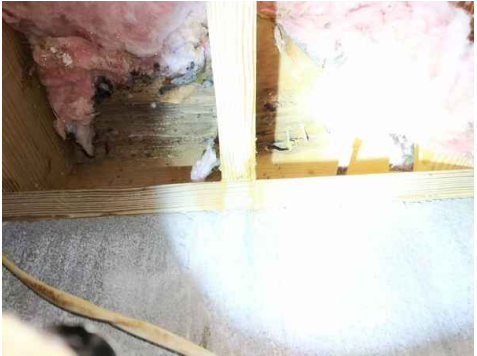
4 - below the front door
